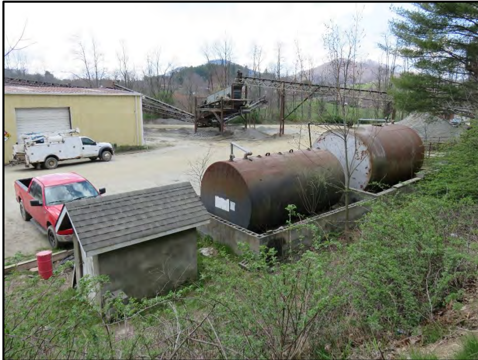
Figure 19: Northwestern view of both tanks and the concrete block shed, looking northwest.
